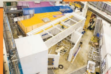
Below: Construction of the Larmor blockhouse next to the other TS-2 reflectometers.
